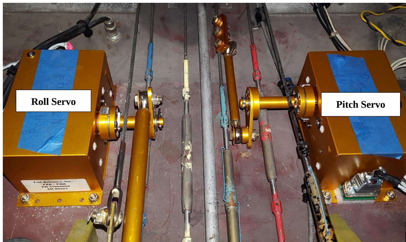
IMAGE 2-2 SERVO INSTALLATIONS GENERAL VIEW
